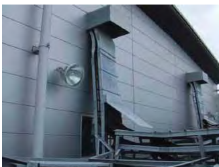
Sharply bent electric wires.
