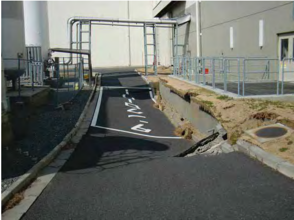
West side road from MLF. About 1.5 m sinking was observed.
