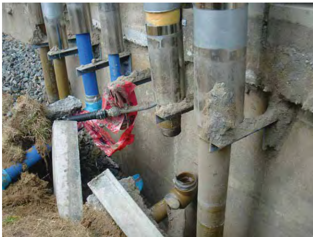
Many pipes were disconnected (upper).
