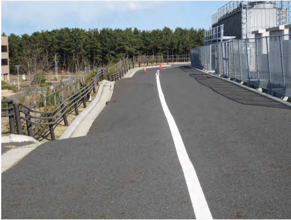
Wavy road. Bump in the middle means that beam pipe is underneath it. Both sides of the bump were sinking.
